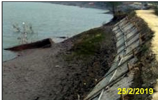
Protective layer Manmathanagar
